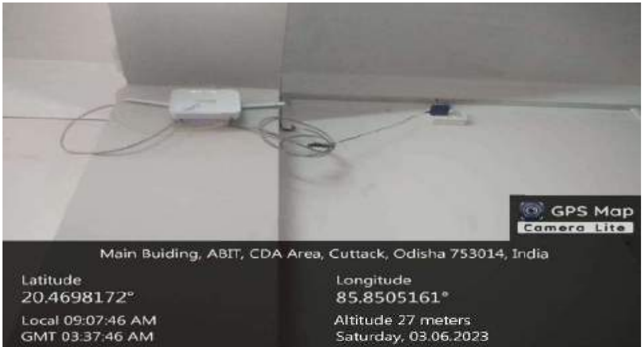
Wi – Fi Access Point
