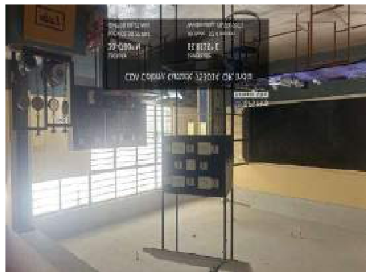
Room No E-103 Energy Conversion Device Lab
